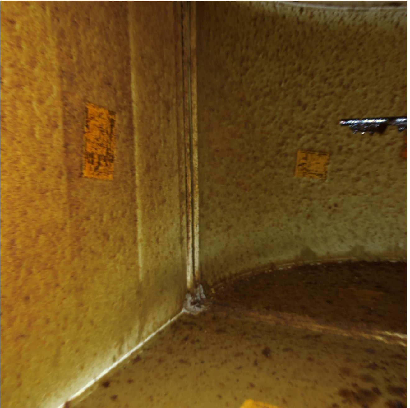
Grill Duct August 2021
