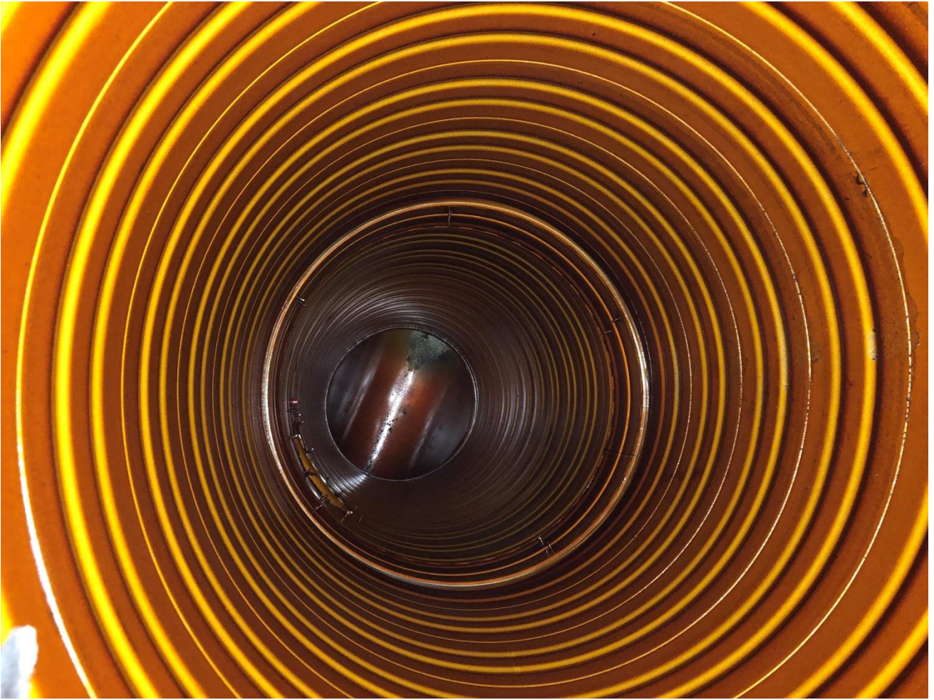
Fryer Duct August 2021
